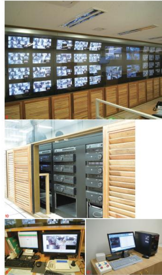
Pic 9,10,11,12 – In Central Monitoring Room of DEP PINO, they can monitor all spots with 80 pcs of monitors and 4 main monitors. 36 pcs of WEBGATE HD-SDI 8ch DVR were installed.
